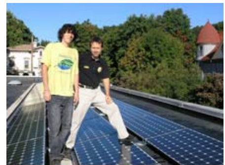
Tsvi Benson-Tilson (left) and Paul Israel of Sunlight Solar on the roof with BEKI's 10.5 kW solar array
